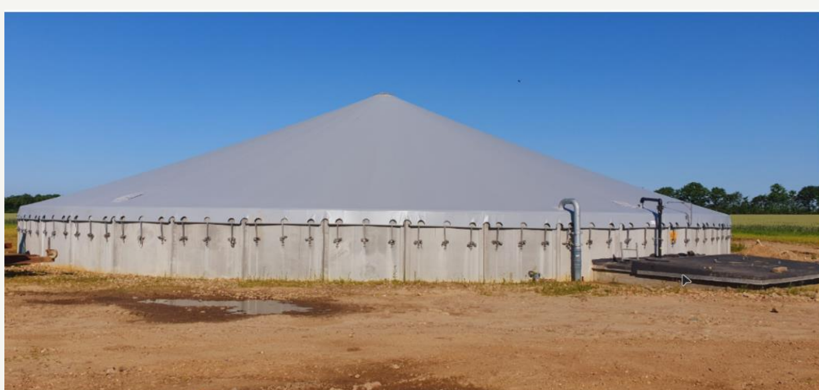
Tank B: Biogas teltoverdækning.
